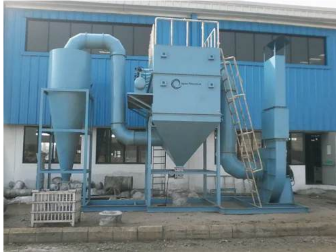
Fig. 2.2.16: Dust collection systems
