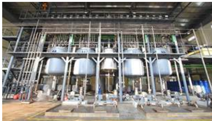
Fig. 10.2.29: Washing and Sanitising Equipment
