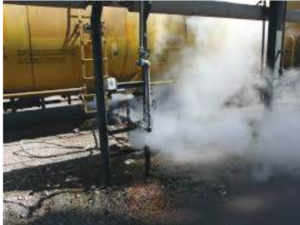
Fig. 2.2.4: Steam or Condensate Leakage during pressing
