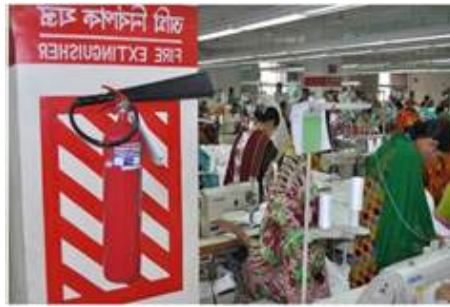
Fig. 6.1.2: Fire extinguishers at the company
